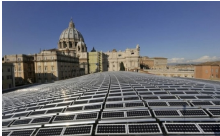
Rooftop solar array in Vatican City. The 2400 photovoltaic panels provide energy for lighting, heating, and air conditioning.
